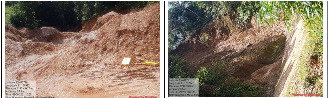
Figure 12: Landslide Prone Location along the project road
